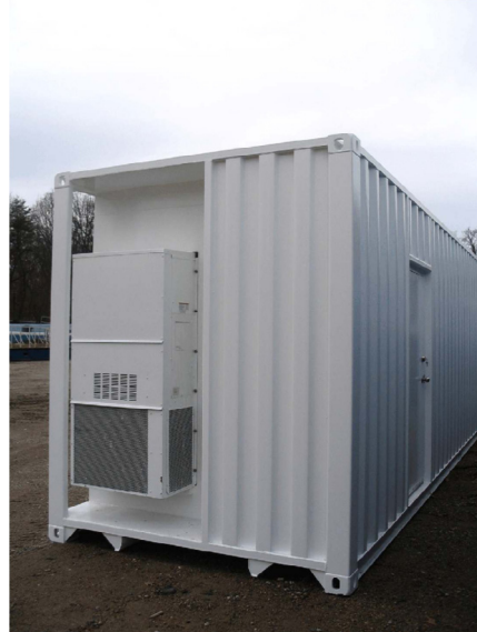
Environment Control (HVAC) and Side Personnel Door for Multiple Access
