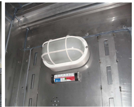
Internal lighting dual voltage source 115/230 VAC
